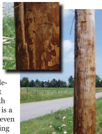
Lightning damage caused to pole where copper ground wire was stolen.
